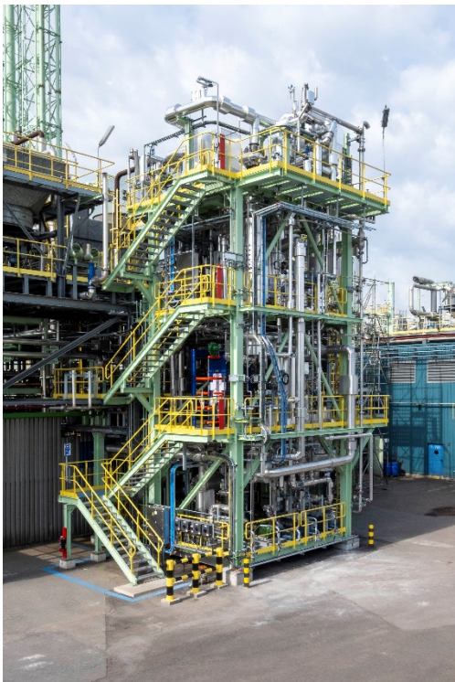
Photo: Start-up of heat recovery unit based on revolutionary Qpinch technology: demonstration unit in Antwerp to test capabilities of technology as well as scale-up potential for wider Borealis operations and technologies.
