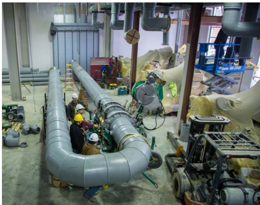
Photo 1 : Fusion welding of large diameter PP-RCT Pipe System for a Chiller Plant
